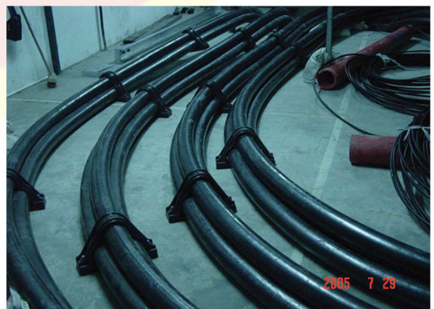
Non-Metallic Trefoil Cable Cleat Silibin 132kV Substation
