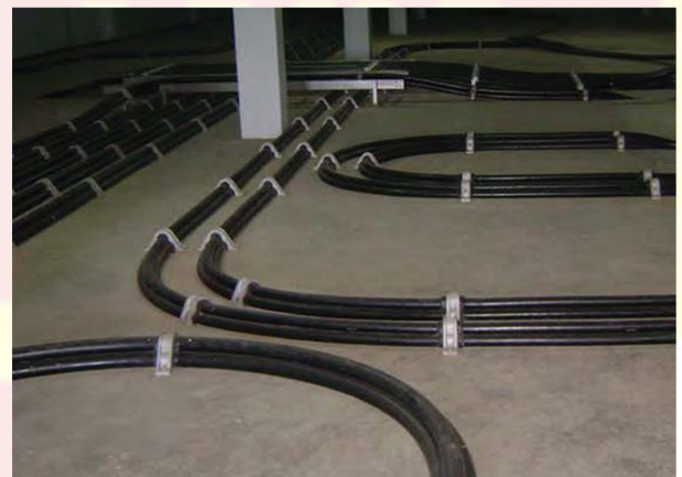
Aluminium Trefoil Cable Cleat Lahat Datu POIC 132kV Substation
